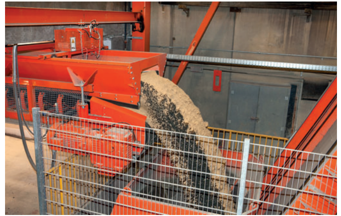
Figure 11: Here, a dry batch is transferred from the weigh belt to the skip hoist prior to loading into the mixer.
