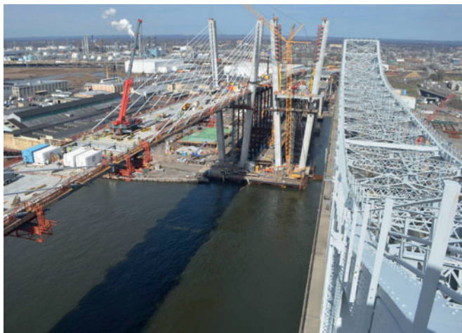
Figure 1 : The twin spans of the new Goethals Bridge are suspended from four towers, and are under construction next to the original 90-year-old bridge (at right), which connects Elizabeth, NJ and Staten Island, NY. [photo courtesy The Port Authority of New York and New Jersey; web cam view March 2017.]
