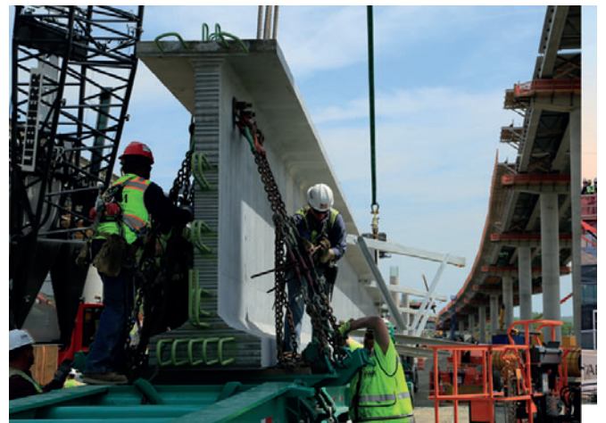
Figure 2: Workers secure one of 400 precast, prestressed bulb-T beams—supplied by Northeast Prestressed Products—to the Goethals Bridge Replacement Project. [photo courtesy The Port Authority of New York and New Jersey]
