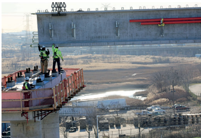
Figure 3: Each 110-ton bulb-T girder is up to 178 feet long, eight feet tall, and three-and-a-half feet wide. [photo courtesy The Port Authority of New York and New Jersey]
